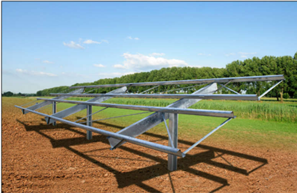
Plate 2-2 Example of a solar PV support structure.
